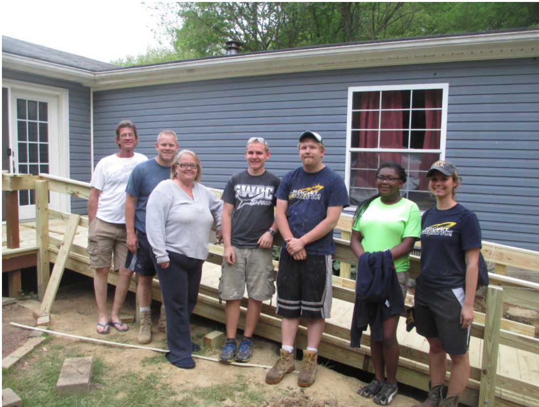
Engineers in Christ after completing the handicapped ramp for Myrtle down in the Appalachia
